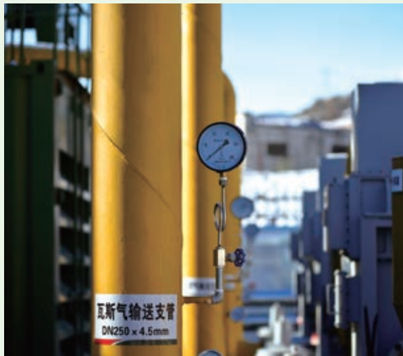
Methane power generation project of Liuhuanggou Coal Mine
